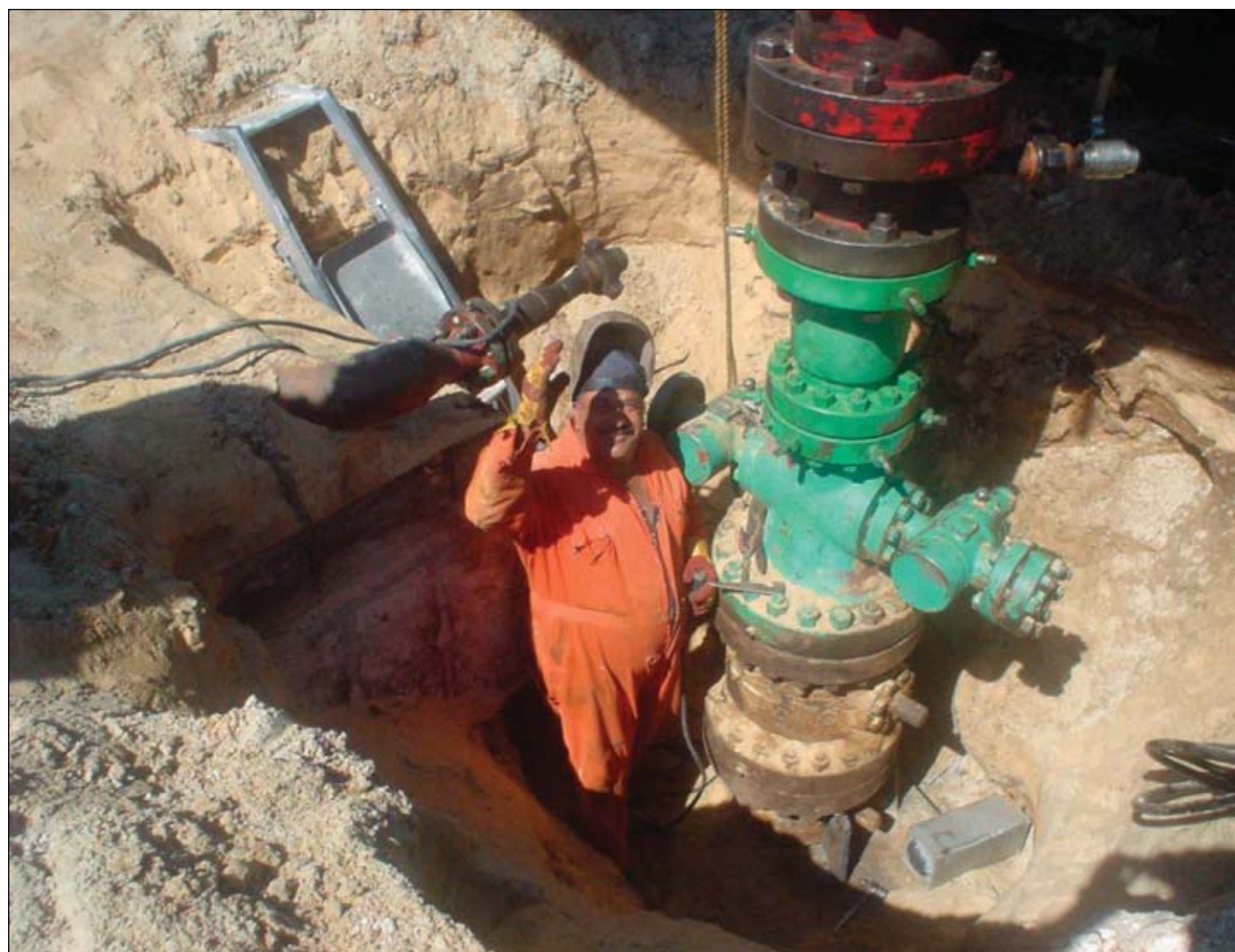
Installation of the baseplate required digging out the cellar to just below Section A (Fig. 3).
